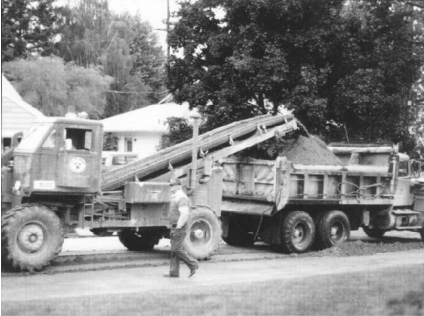
FIGURE 4.1. Clean-up operations after only 1 centimetre of ash fall in Yakima, USA, following the 1980 Mt St Helens eruption (photo City of Yakima).
